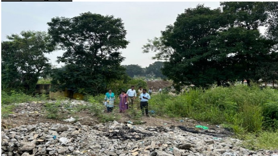
Dumping of Debris and C&D waste observed
